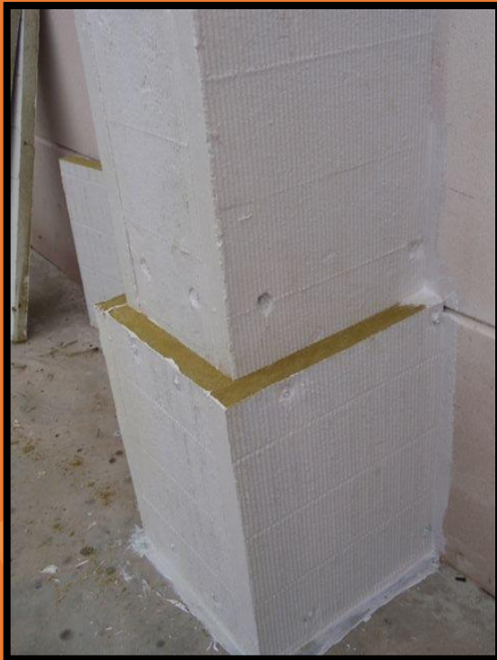
Three sided vertical riser shown in image above
